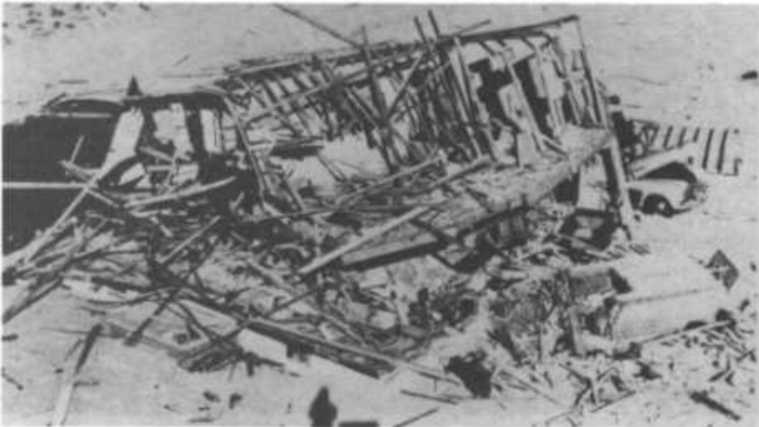
Fig. 7.4. Unburned wreckage of the same two-story, wood-frame house pictured in Fig. 7.1 after being wrecked by the 5-psi blast effects of a small nuclear test explosion.
